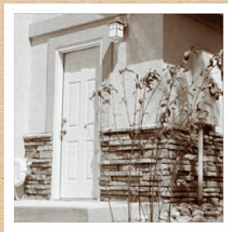
Stone wainscot extends close to the ground while wrapping the corner and terminating at wall plane change.
